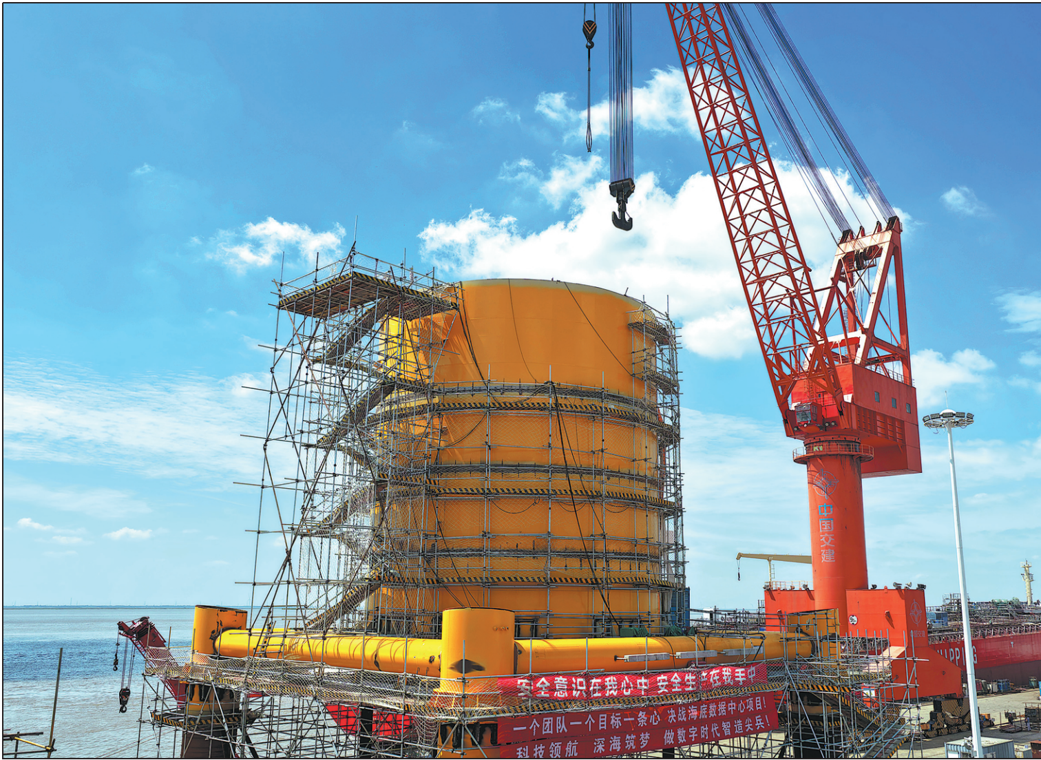
A photo shows the data cabin of the Shanghai Lingang undersea data center demonstration project on Sept 11. XU CONGJUN / FOR CHINA DAILY
