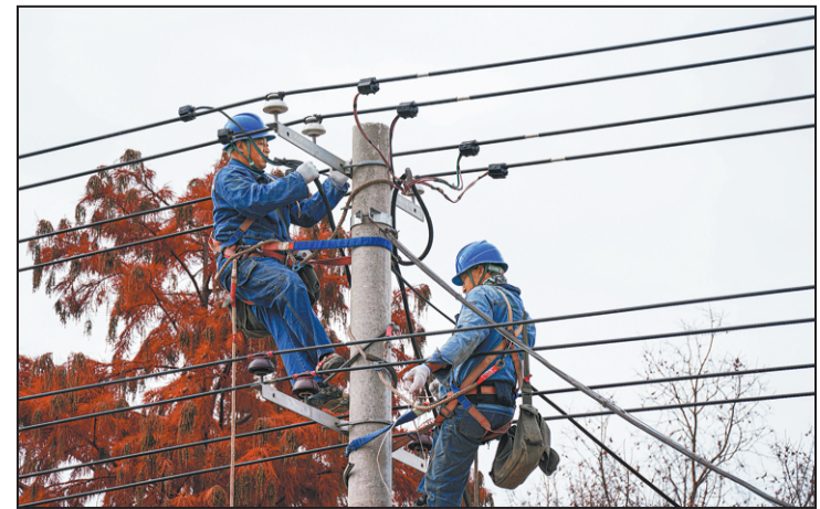
Employees from State Grid Hefei in Anhui province carry out low-voltage treatment work in Suwan town in Chaohu, providing a solid guarantee for rural electricity supply in the winter.
