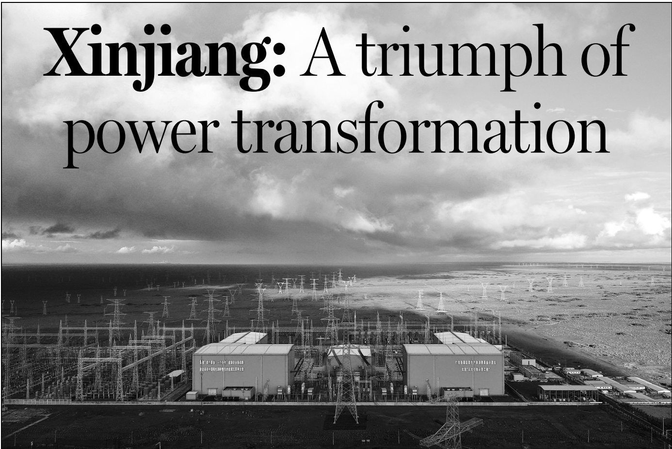
Changji converter station is seen in the barren land of Changji Hui autonomous prefecture, Xinjiang. PROVIDED TO CHINA DAILY
