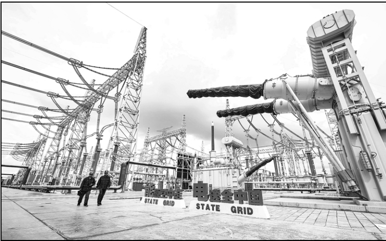
Middle: Workers inspect equipment at the Changji converter station, the beginning of the Changji-Guquan Ultra-High-Voltage Direct Current Transmission Project. HE LONG / FOR CHINA DAILY
